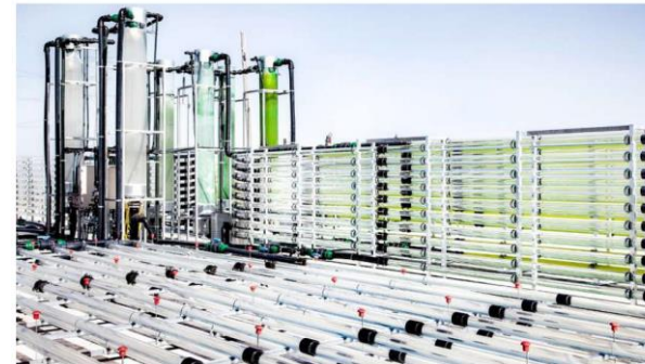
Details for Tubular bioreactors filled with green algae fixing CO2
